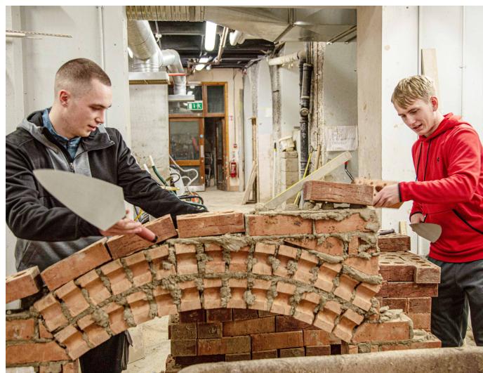
Bricklaying apprentices Jack Grehan and Gary Kett working on a brick arch at the Bolton Street College Training Centre in Dublin.
